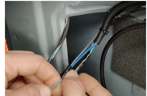
Connecting M1 Wires
